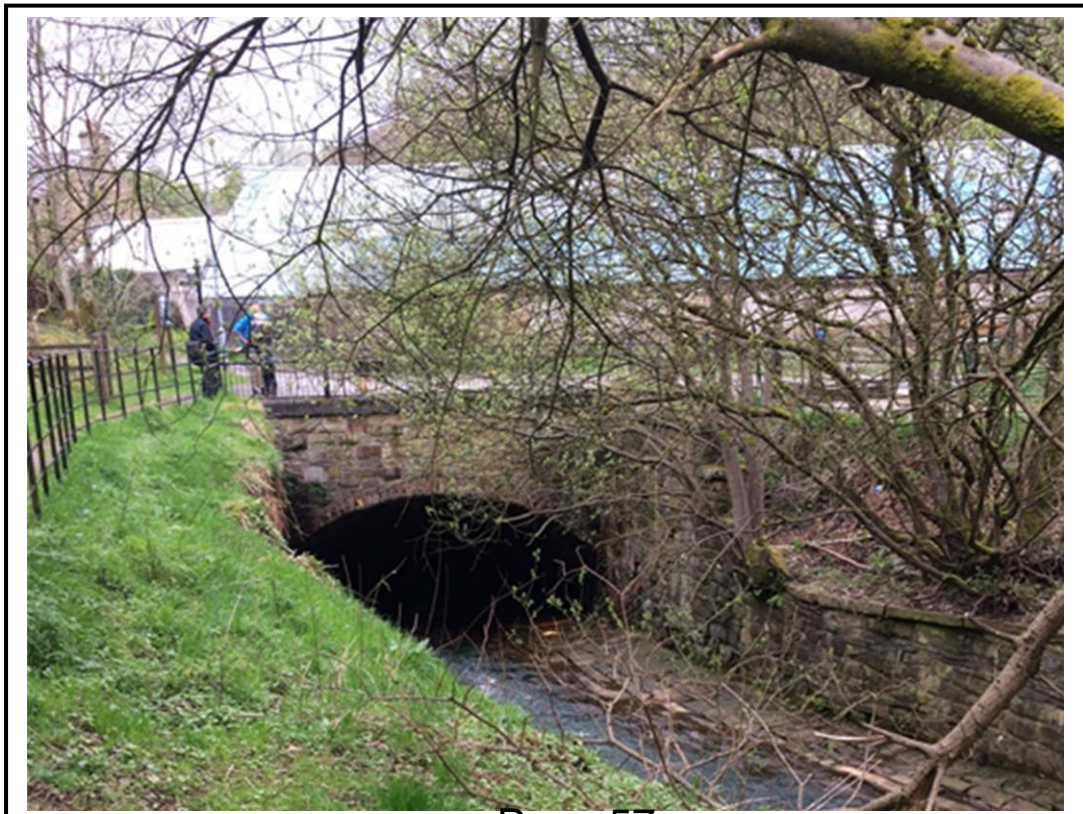
Photo 6 – view towards the southern edge of the site, with the bridge over the River Medway on Mill Brow in the foreground.
